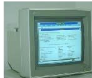
Total Control System
